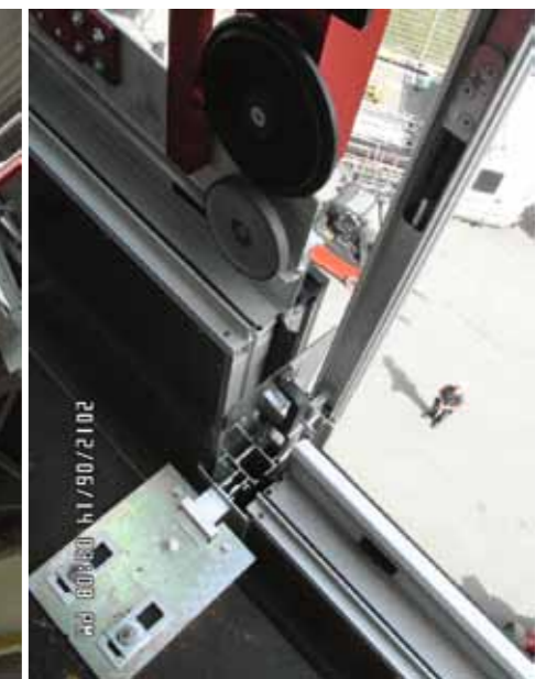
A façade element is placed on the brackets automatically, and is driven by its own weight
