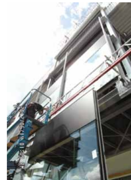
A façade element is fixed in the lifting profile and moved upwards
